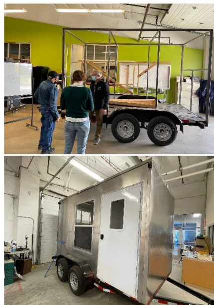
Figure 3: The construction of the Sunchaser2k22 is seen here from its initial framing to near completion
