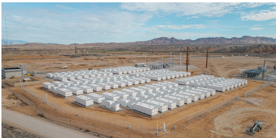
The Reid Gardner Battery Energy Storage project near Moapa, Nevada | Source: Wikimedia Commons
