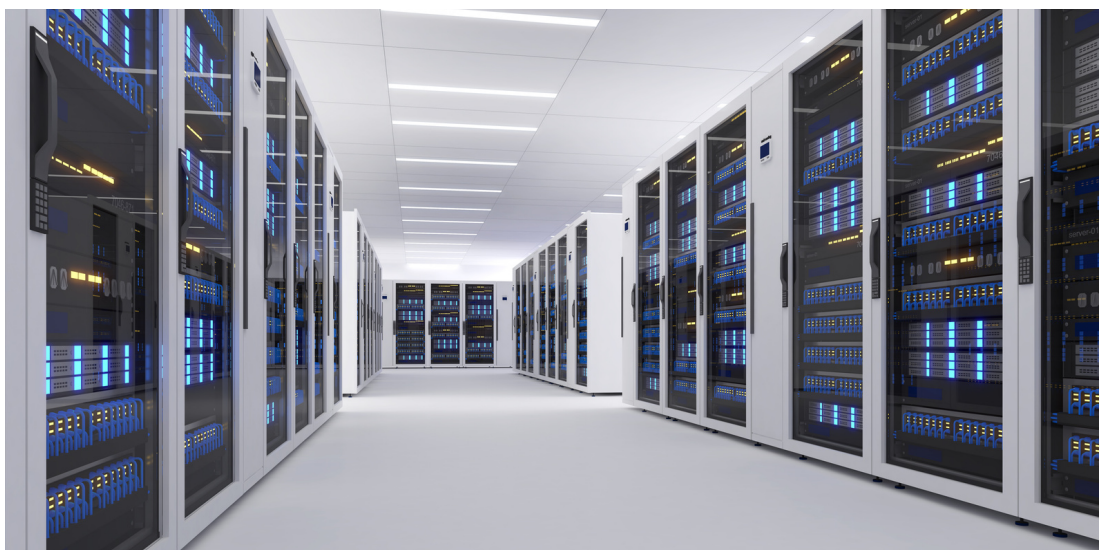
Photo of a data center | Source: Canva
